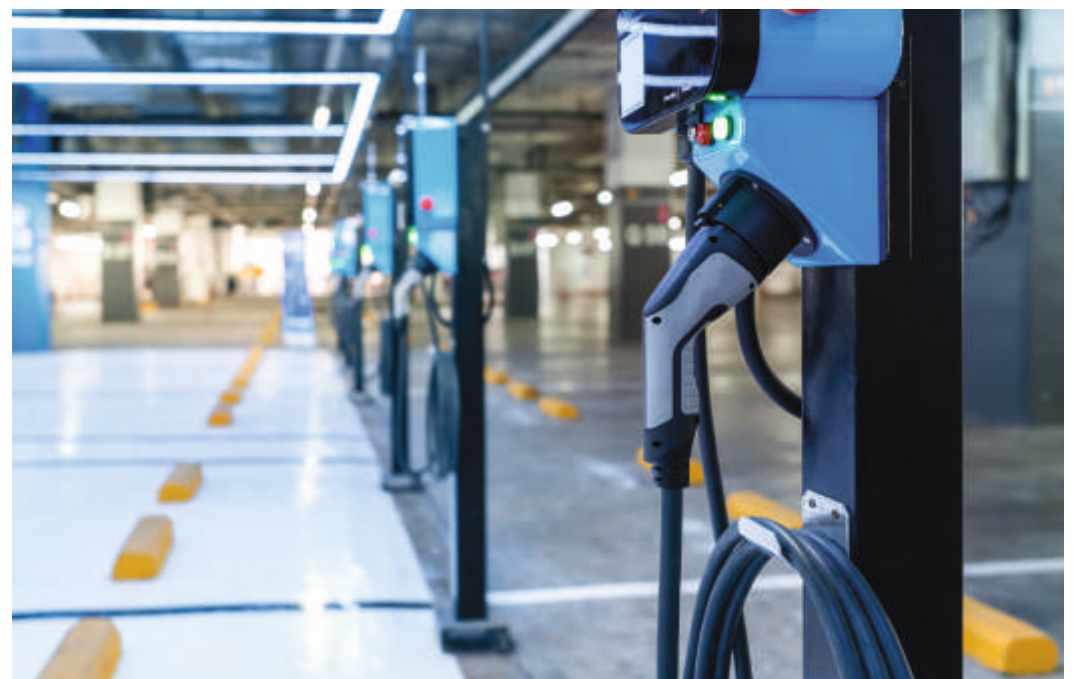
EV Charging Station
